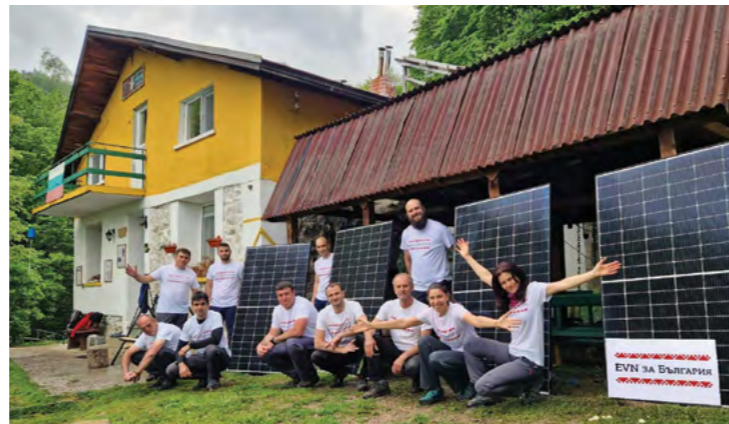
The volunteers installed rooftop solar panels on the Ravnets hut in Stara Planina.
